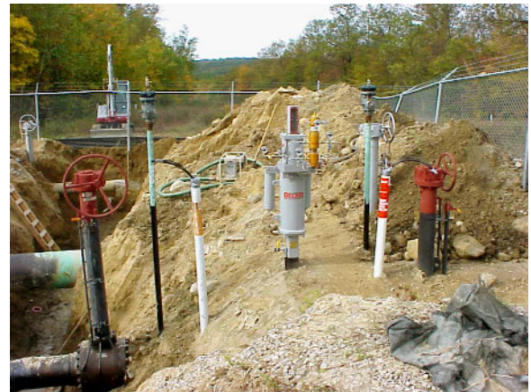
Figure 11.0 – Becker Below Ground Monitor Valve Becker Model VRP-600-SB-CH pilot installed on a fail-closed Becker RPSR series actuator used as over-pressure protection. The Becker FPCV-T0 Control Valve is buried for noise attenuation.
