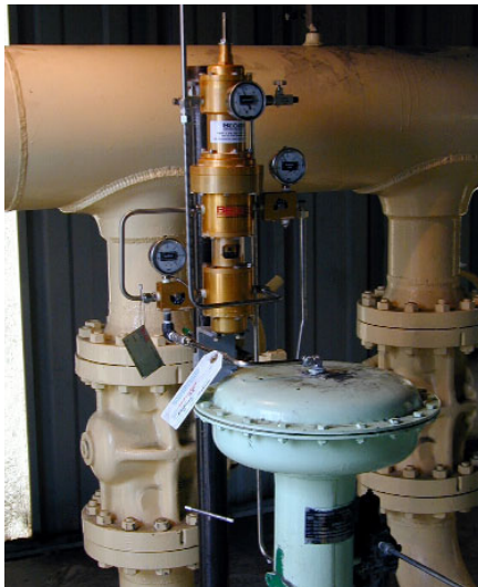
Figure 8.0 - VRP-SB-CH Retrofit Simplifies Control Instrumentation
